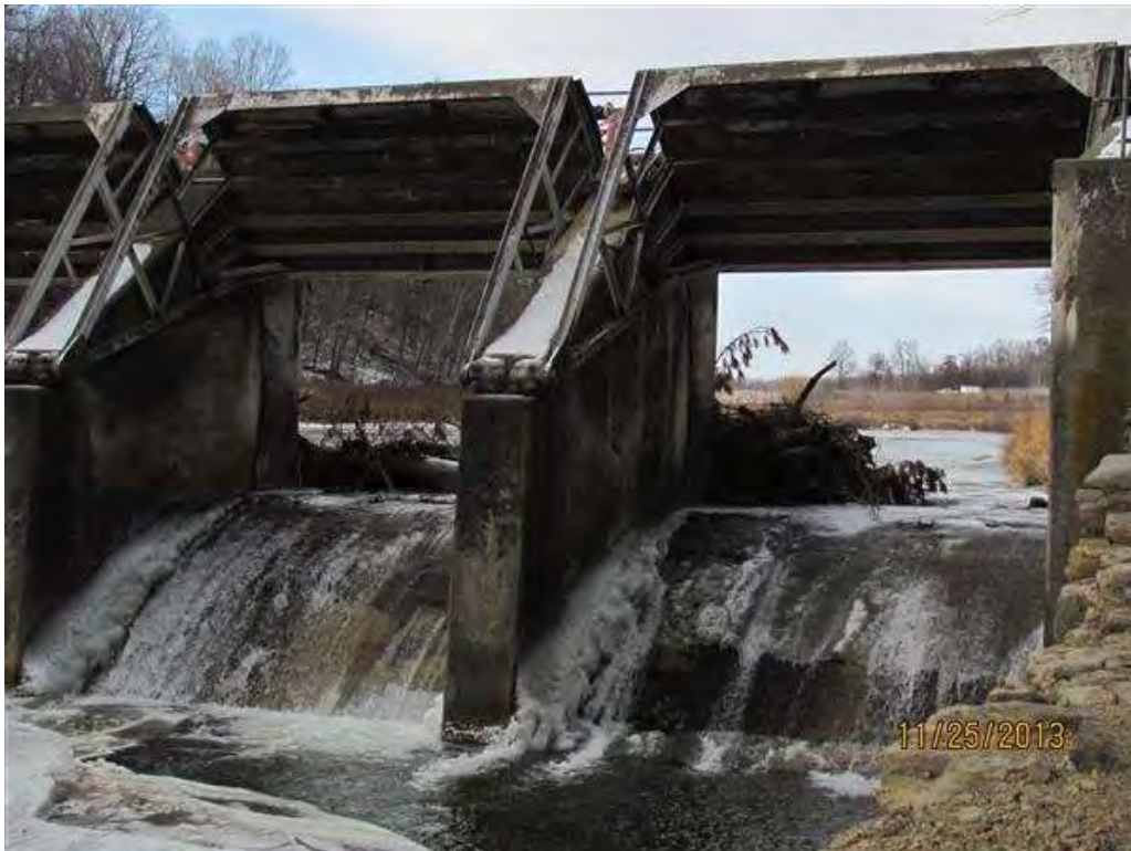
Photo 10 - Timber debris at dam.
