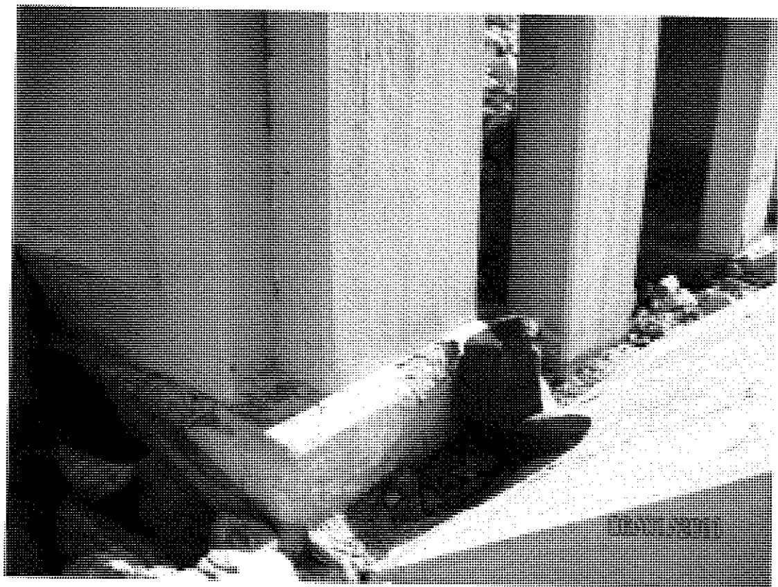
Photo 8 - West Arch Column 1 North End
