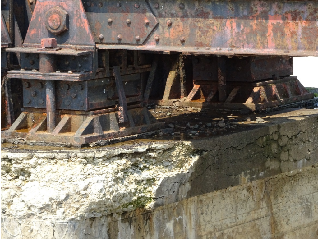
Figure 5-15 Photograph of Bridge 49553 Pier Cap Concrete Deterioration.
