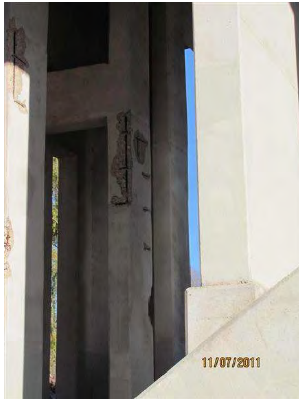
Photo 3 - North Columns spalls
