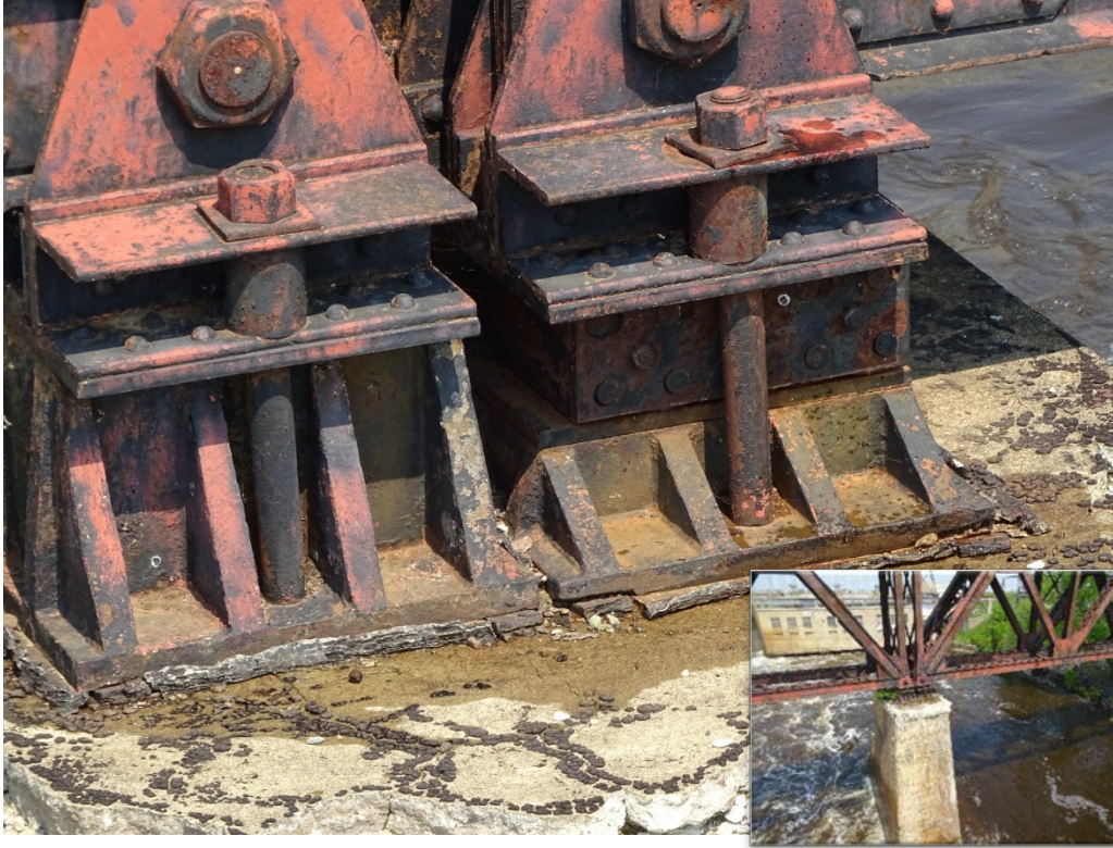
Figure 3-3 Example of the Detail Obtained at a Difficult to Access Bearing Location.
