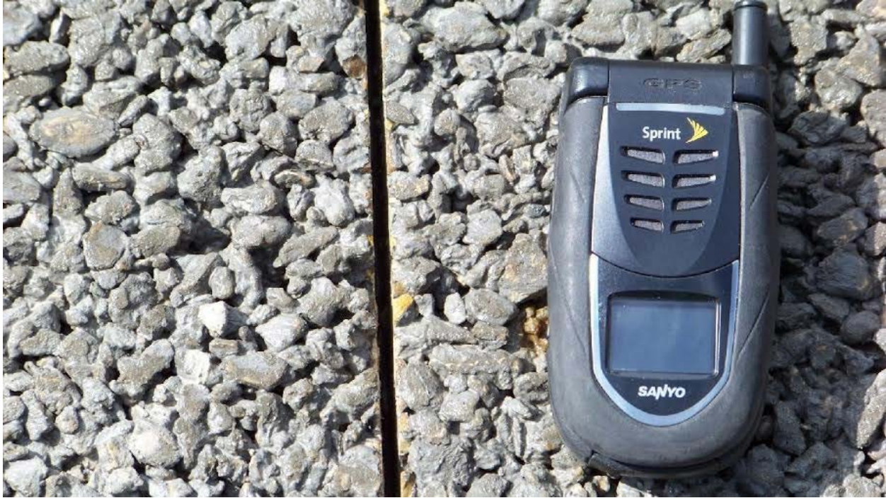
Figure 9.15. Saw cut joint in pervious concrete at Woodbridge neighborhood, Shoreview, MN (photo courtesy of M. Maloney, City of Shoreview).
