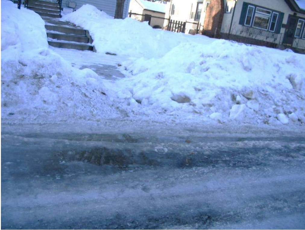
Figure 9.13. Slush gathering and refreezing on the traditional asphalt at Site 1 on January 17, 2010 (Wenck 2014).
