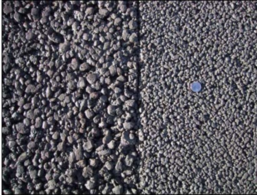
Figure 9.26. Pervious concrete at Lakewood City Shops maintenance building. AASHTO #67 mix is on the left and AASHTO #8 is on the right (UDFCD 2011a). A quarter is placed on the AASHTO #8 pavement for scale.
