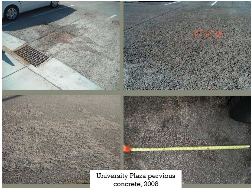
Figure 9.22. University Plaza pervious concrete parking lot in 2008 (photo courtesy of K. MacKenzie, UDFCD).
