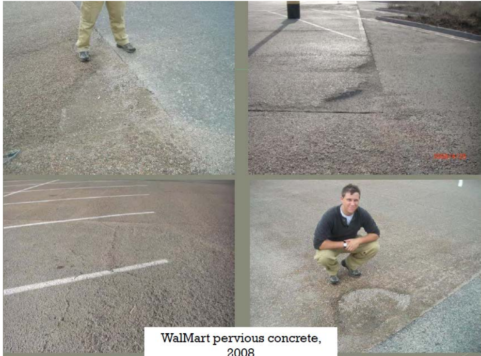
Figure 9.20. Aurora Wal-Mart pervious concrete parking lot in 2008 (photo courtesy of K. MacKenzie, UDFCD).
