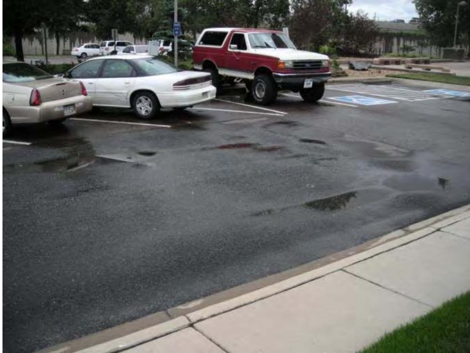
Figure 9.25. Porous asphalt pavement at Denver Waste Management building after a light rain (photo courtesy of K. MacKenzie, UDFCD).
