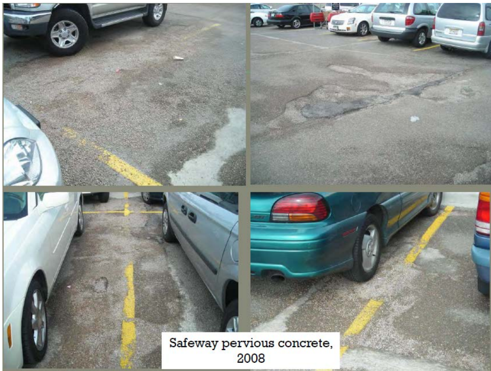
Figure 9.21. Denver Safeway pervious concrete parking lot in 2008 (photo courtesy of K. MacKenzie, UDFCD).
