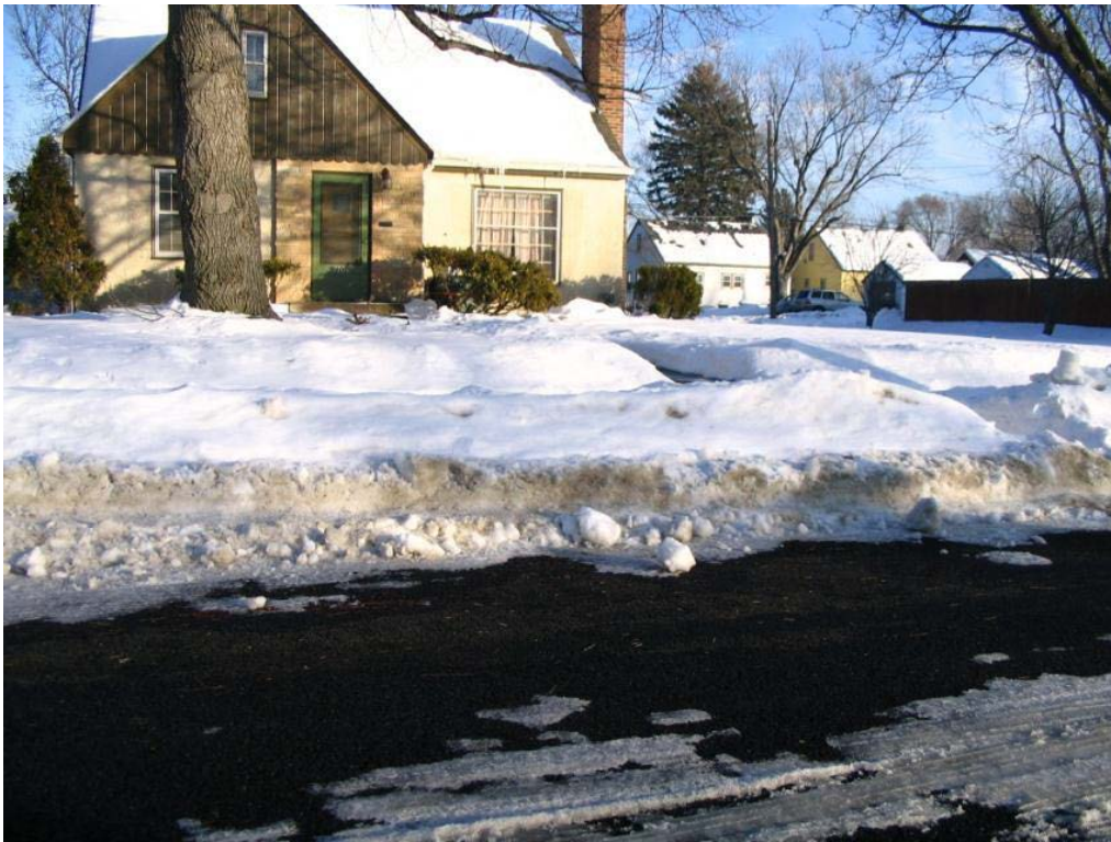
Figure 9.14. Slush free porous asphalt on January 17, 2010 (Wenck 2014).
