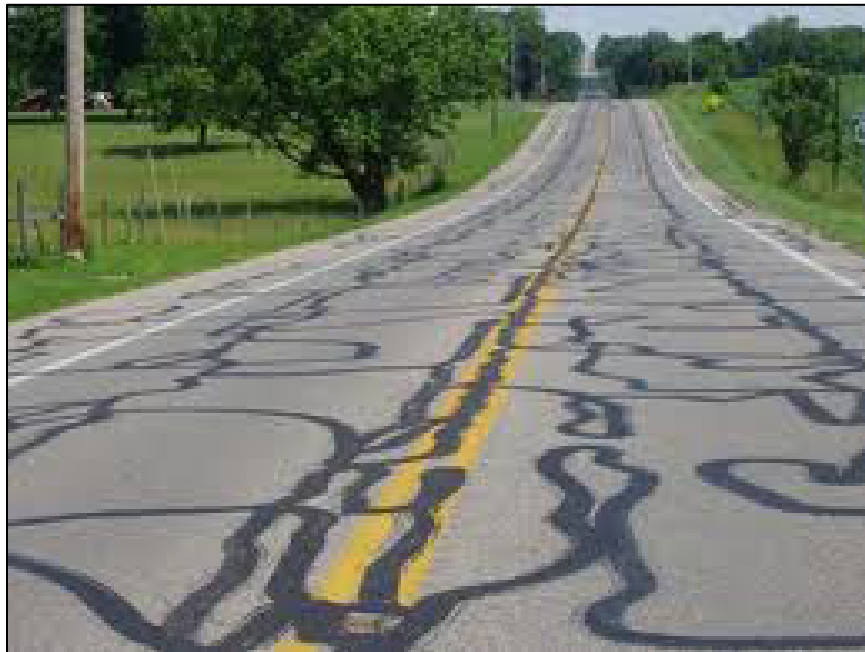
Figure 14. Not a good candidate for pavement preservation activities.
