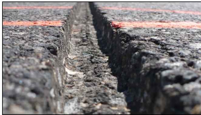
Figure 24. A clean, dry, routed crack.
