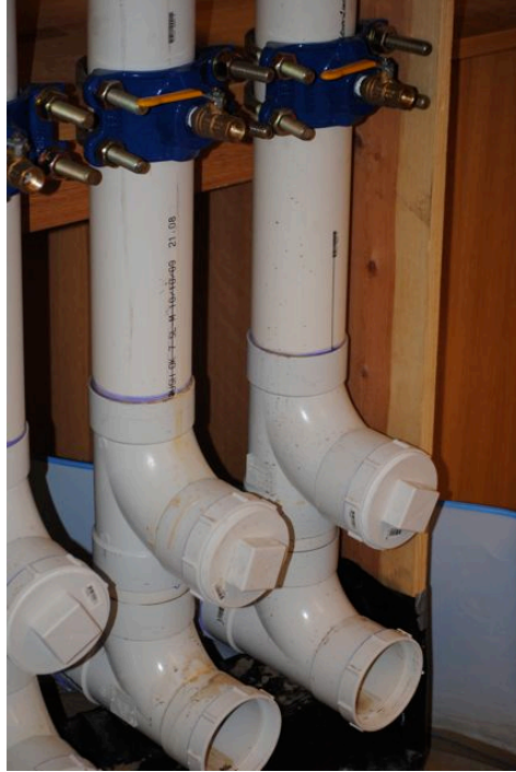
Figure 11. Sedimentation columns. Only bottom third of each 8-foot column shown, with 6-foot depth valved sampling port (attached to blue saddle tap) and two sludge clean outs. Open top and 2-foot and 4-foot depth valved sampling ports not shown.
