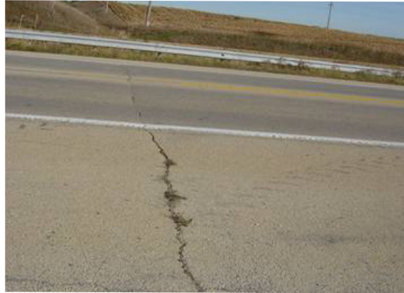
Low-temperature cracking (transverse cracks) may occur when asphalt pavements contract in cold temperatures.
