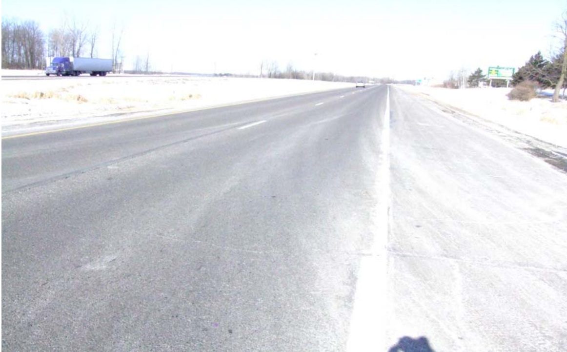
Figure 9: Transverse Cracks Reflecting Through the UTBWC Overlay. Photo Taken at RP 183 NB on February 14 th , 2007.
