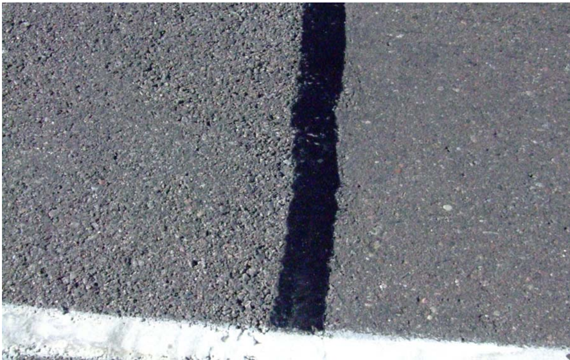
Figure 10: UTBWC Pavement Located on the Left and Control Section on the Right- February 14 th , 2007.
