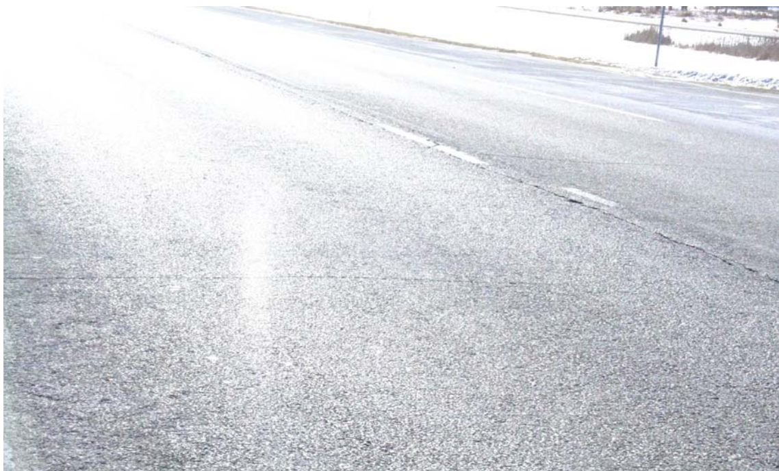
Figure 8: Transverse Cracks Reflecting Through the UTBWC Overlay. Photo Taken at RP 183.5 NB on February 14 th , 2007.
