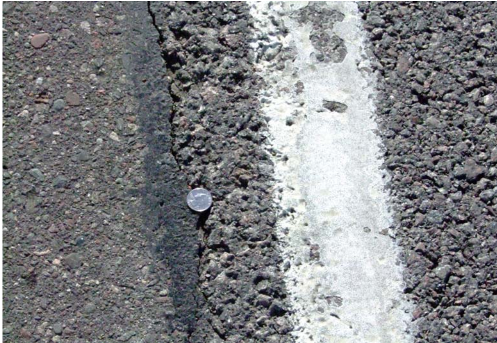
Figure 7: Longitudinal Edge Crack - after 7 years. Photo Taken at RP 184 NB on February 14 th , 2007.
