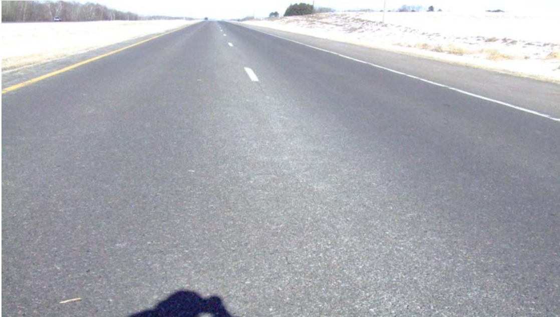
Figure 5: UTBWC Overlay Section (Paved in August 2000). Photo taken at RP 181.00 NB on February 14 th , 2007
