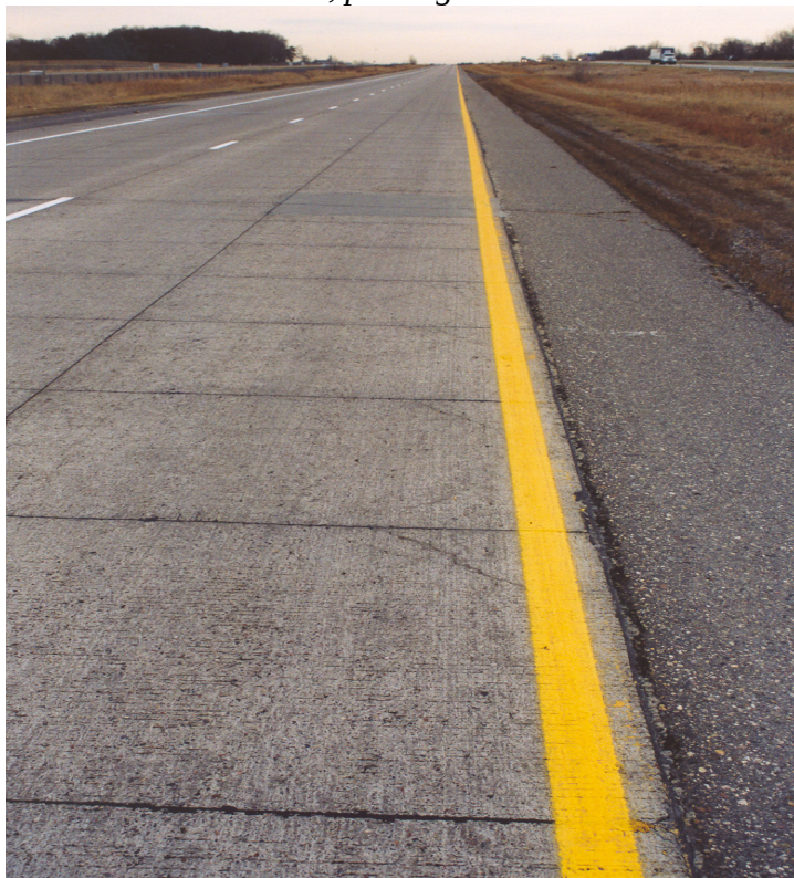
Photo 2.11. Corner cracking on the outside edge of panels near the shoulder, November 2003. MnROAD Test Cell 95, passing lane.
