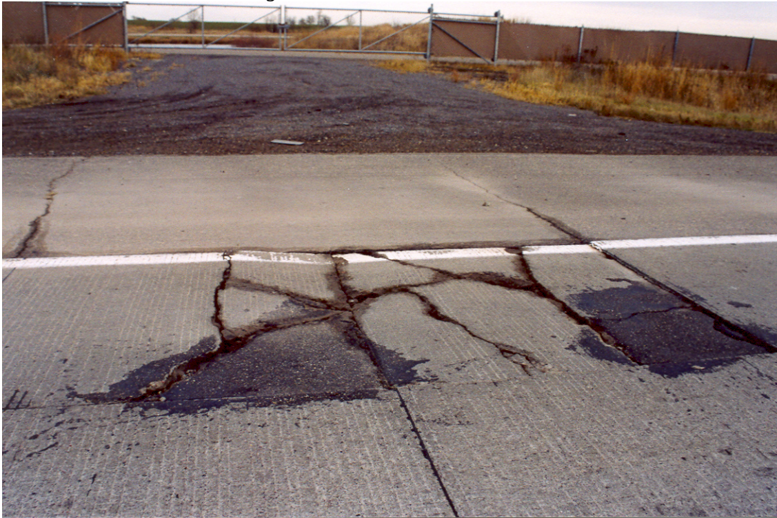
Photo 2.6. Load related cracking and large surface depression, November 2003. MnROAD Test Cell 93, driving lane.
