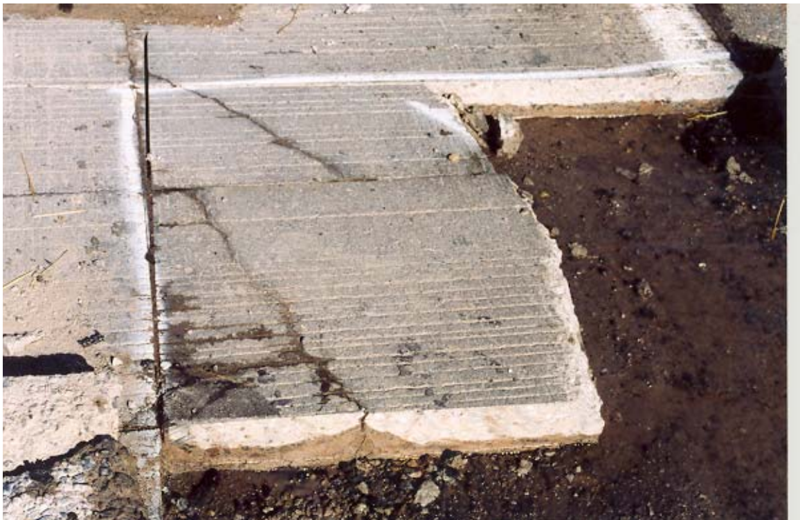
FA "A", Cell 93 Remaining portions of slab still bonded to HMA. 8-25-2004/B-33
