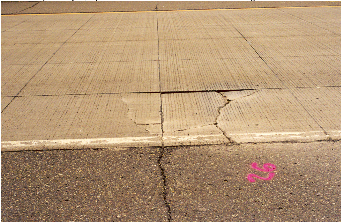
Photo 2.5. Load related cracking and surface depression (punchout) near existing transverse crack in asphalt layer, April 2001. MnROAD Test Cell 93, driving lane.
