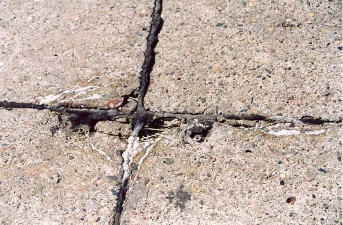
Cell 95 Joint cracking near joint 2155.
