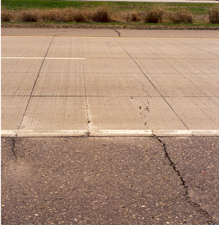
Photo 2.4. Cracks from underlying asphalt layer reflected through UTW overlay, April 2001. MnROAD Test Cell 93, driving lane.
