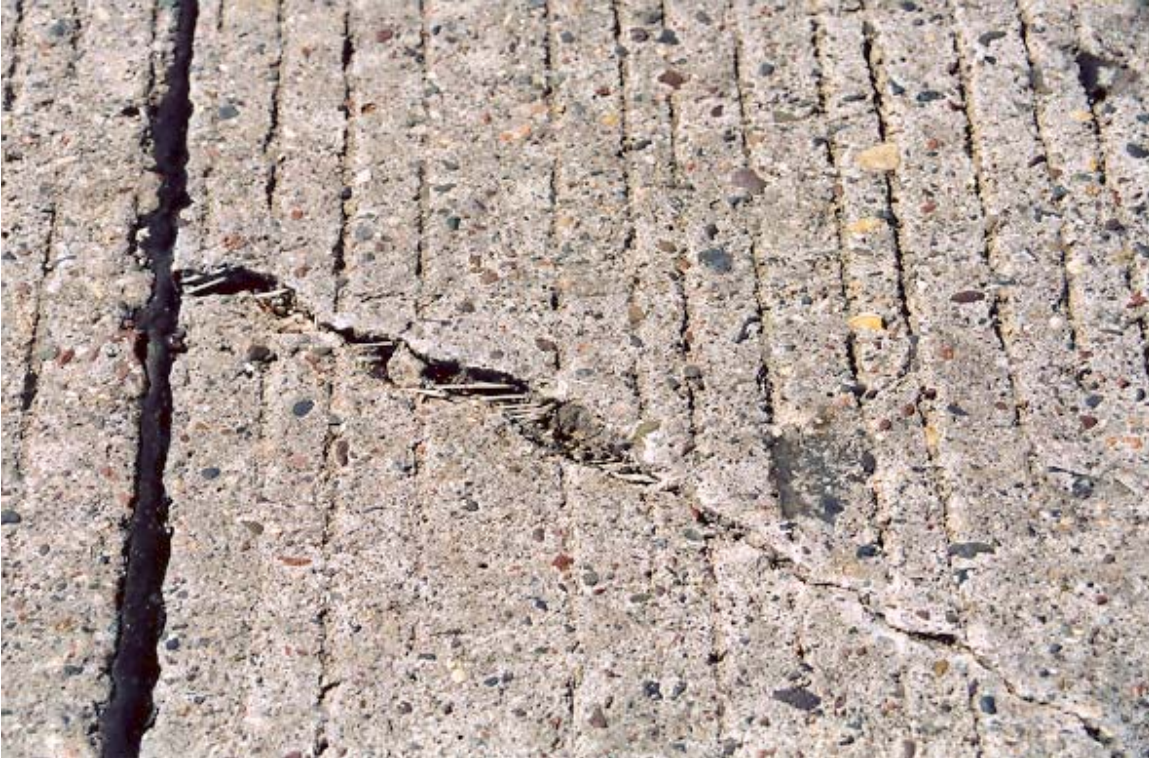
Cell 95 Corner crack near joint 2155.
