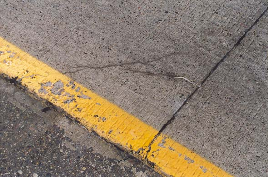
Cell 95 Initial approach panel cracking in passing lane.
