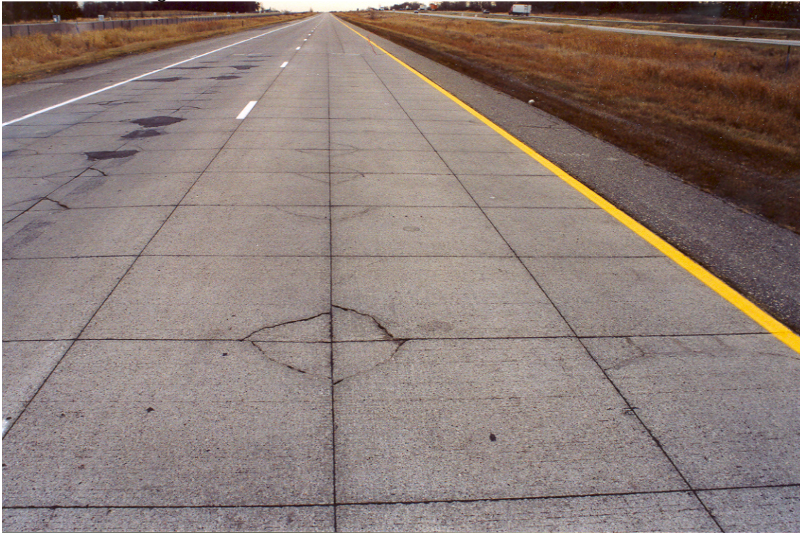
Photo 2.9. Passing lane of test cell 94, beginning to show similar corner cracking distress as driving lane, November 2003.
