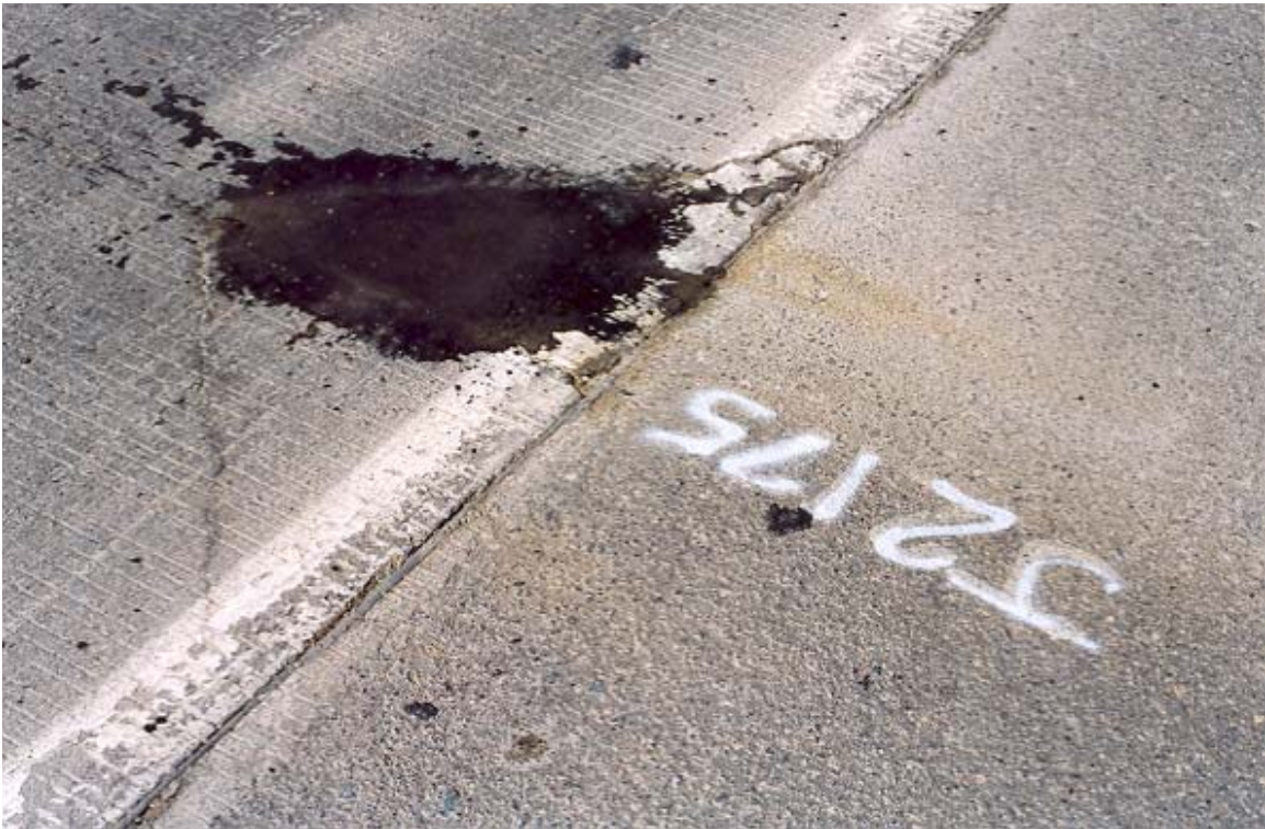
Cell 95 corner crack forming into “pothole”.
