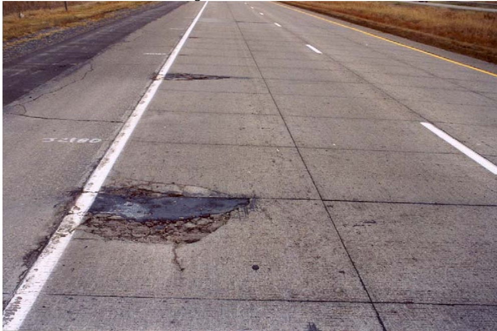
Photo 2.10. Corner cracking on the outside edge of panels near the shoulder, November 2003. MnROAD Test Cell 95, driving lane.
