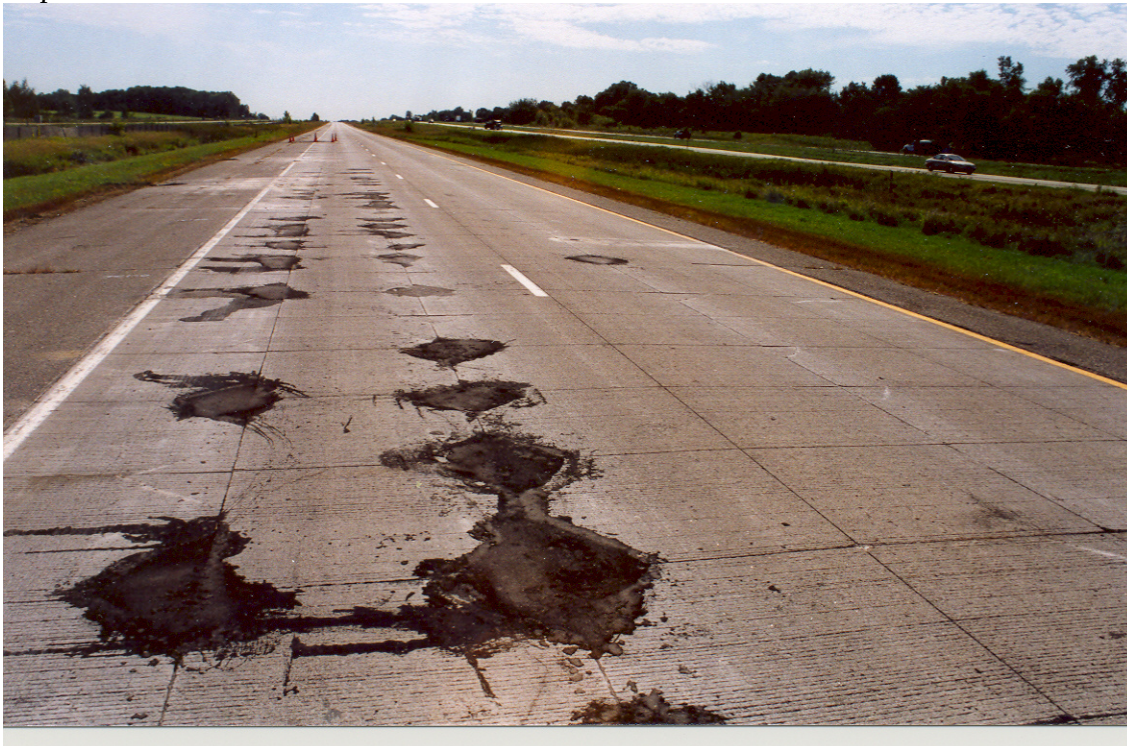
Photo 2.8. Asphalt patching on nearly every panel in the driving lane of test cell 94, September 2004.
