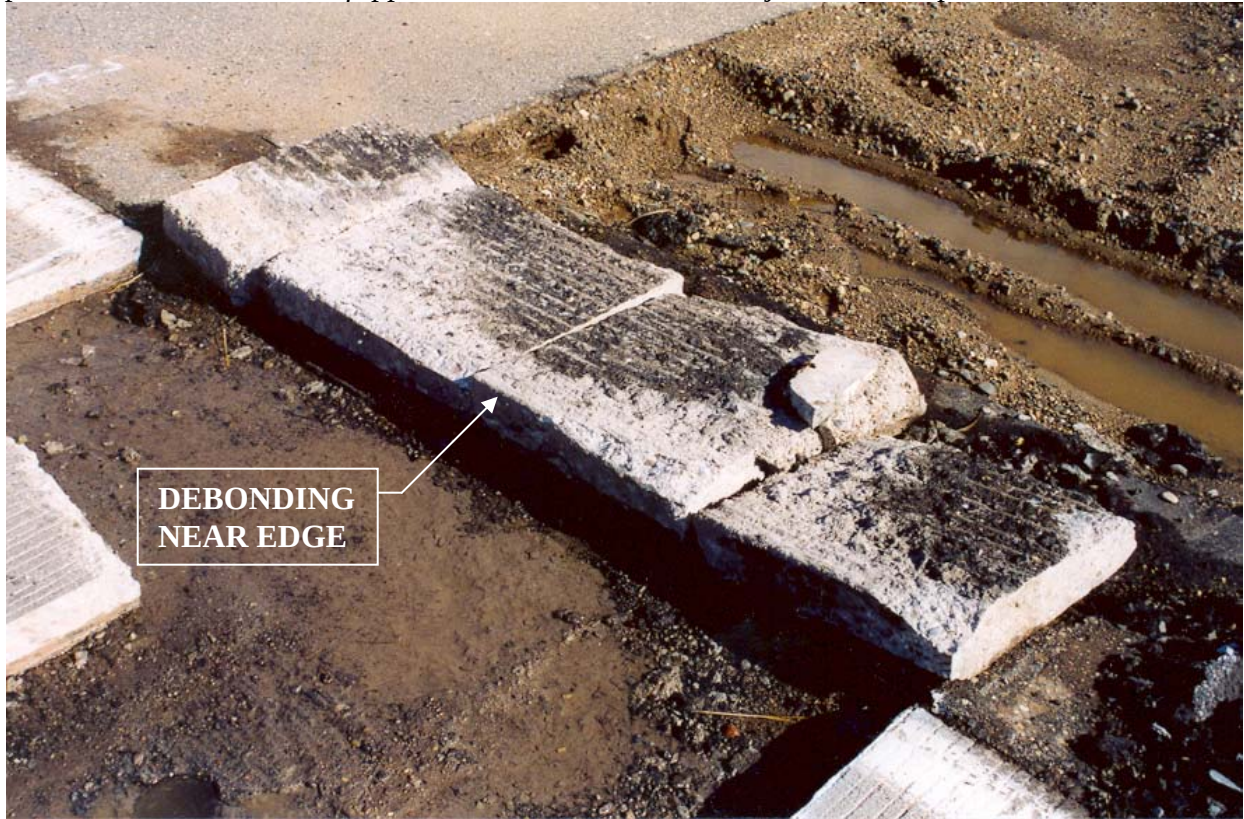
Photo 3.12 Test pit “A” samples showing an area of debonding near the shoulder edge of the panels. Pieces are shown flipped over in shoulder area, adjacent to test pit.
