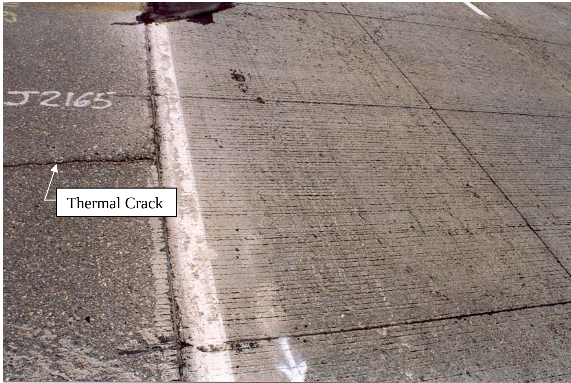
Photo 3.18 Major preexisting thermal crack in HMA that did not reflect through UTW in Cell 95.
