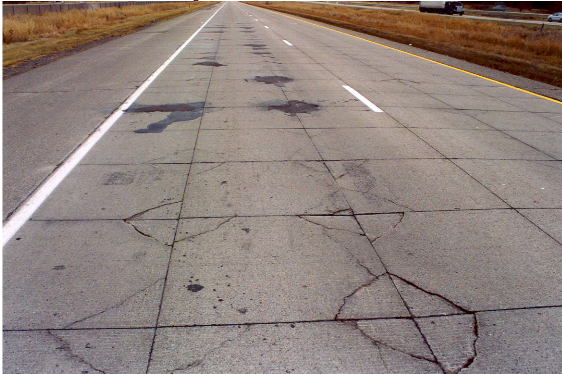
Photo 2.1. Corner cracked areas beginning to punch through the surface in November 2003. MnROAD Test Cell 94, driving lane.
