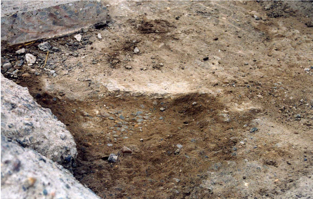
Photo 3.15 Forensic Area “A” showing deformation in HMA from punchout in UTW.
