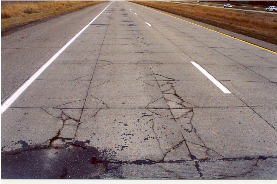
Photo 2.7. Extensive corner cracking on edges of center panels (wheelpaths), beginning to connect to one another, November 2003. MnROAD Test Cell 94, driving lane.
