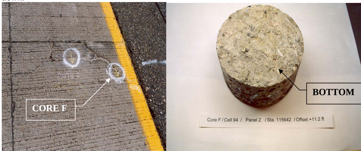
Photo 3.9 Core sample “F” showing no bond between UTW and HMA. Core shown upside down.
