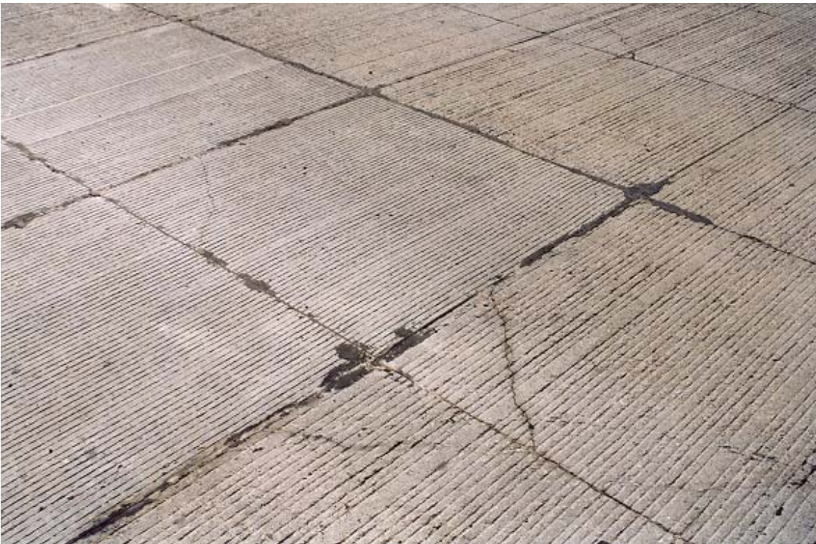
Cell 94 Early corner cracking on inside wheelpath of driving lane.
