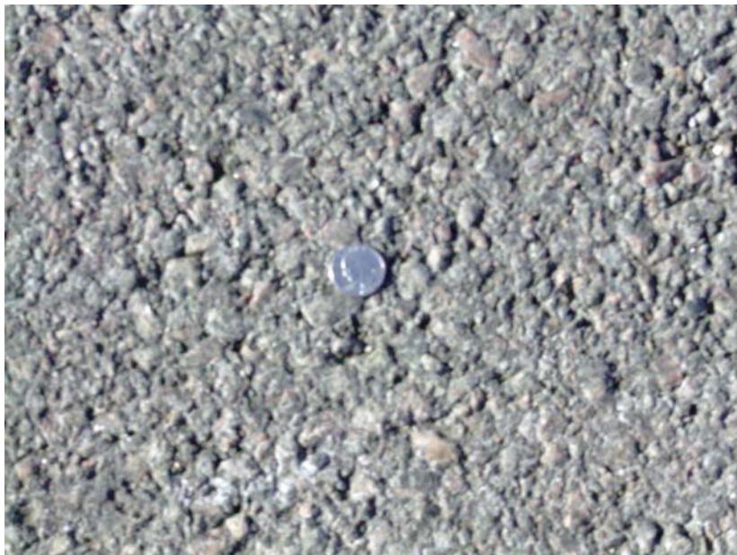
Figure 1: Texture of UTBWC on US-169. Photo Taken at RP 182 NB on February 14 th , 2007. UTBWC was placed in August 2000.
