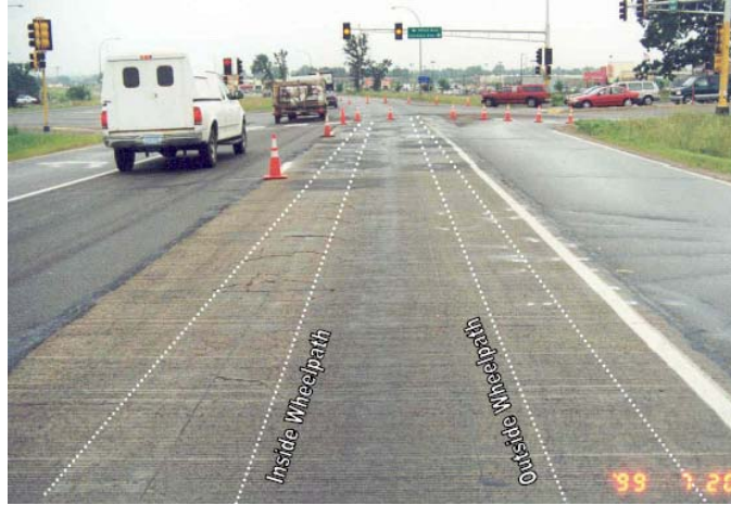
Figure 5.2 Corner Breaks in the Wheelpath at Jackson St. Sections on US-169, Elk River
