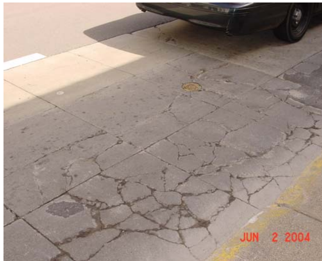
Figure 5.5 Shattered Bus Pads in Downtown St. Paul
