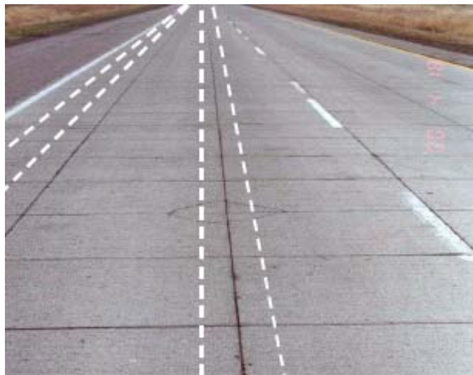
Figure 5.4 Corner Breaks on I-94
