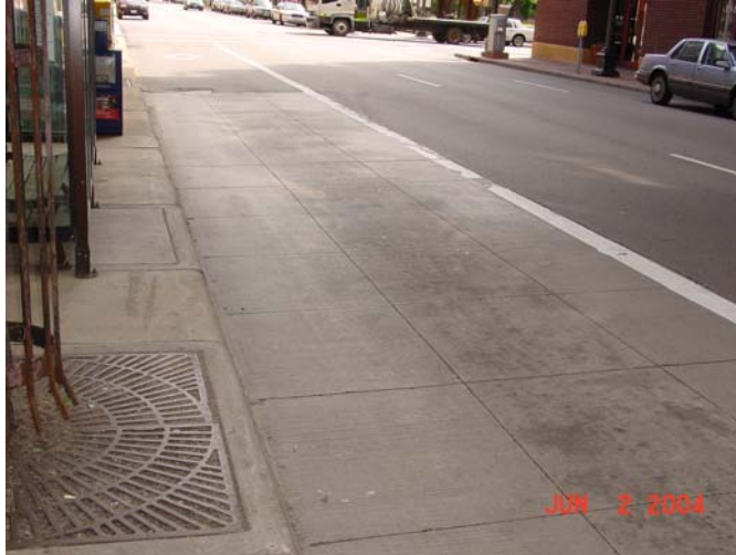
Figure 5.6 Intact Bus Pads in Downtown St. Paul
