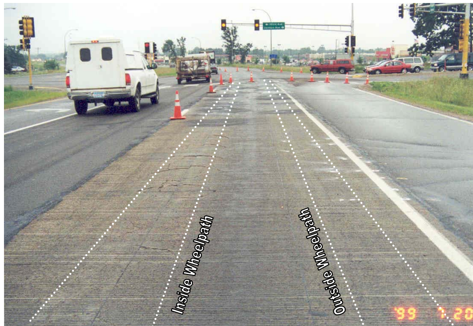
Figure 4.2. Corner breaks in the inside wheelpath at the Jackson Street test section (photo was taken on 07.20.99).
