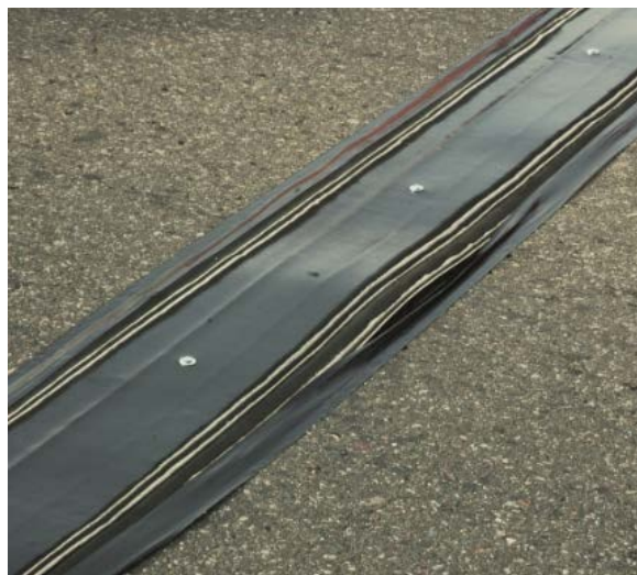
Figure 6: Improperly Installed Weigh-Pad
