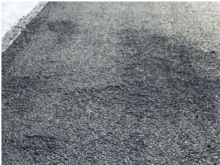
Figure 5.10. Surface raveling, cell 88
