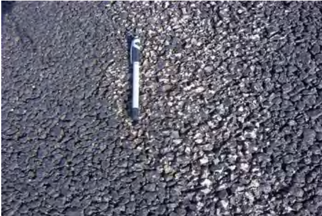
Figure 5.11. Minor snowplow scuffing, cell 86
