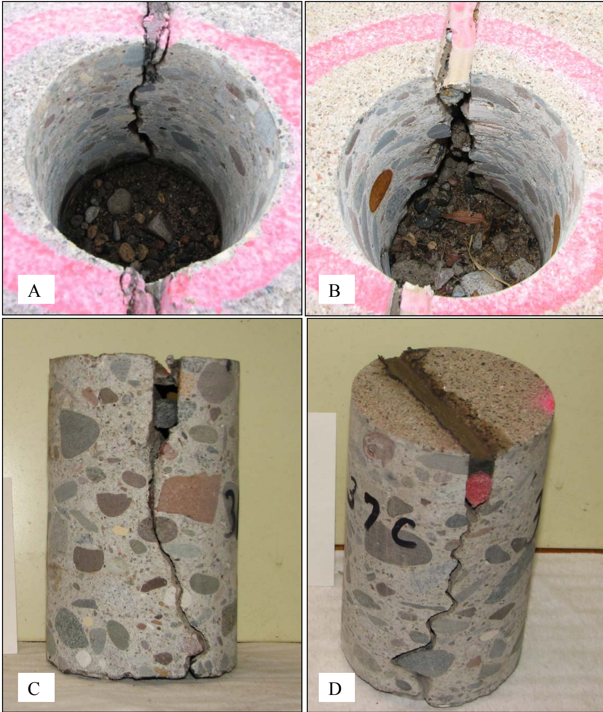
FIGURE 6 A) Core hole from cell 32, a 5 inch JPCP with Class 1 base; B) core hole from cell 36 where joint sealant was in poor condition; C) core from cell 36 where joint sealant was in good condition; D) core from cell 37 where joint sealant was in good condition.
