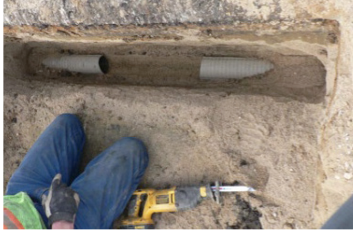
Researchers cut out sections of edge drain pipes to evaluate sediment composition.
