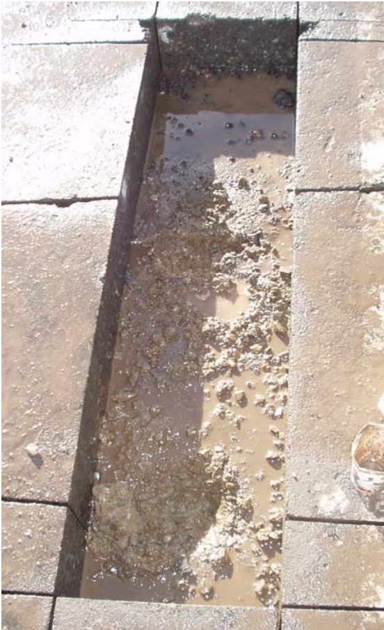
Figure 15 Mn/DOT D1 test pit over saw cut.
