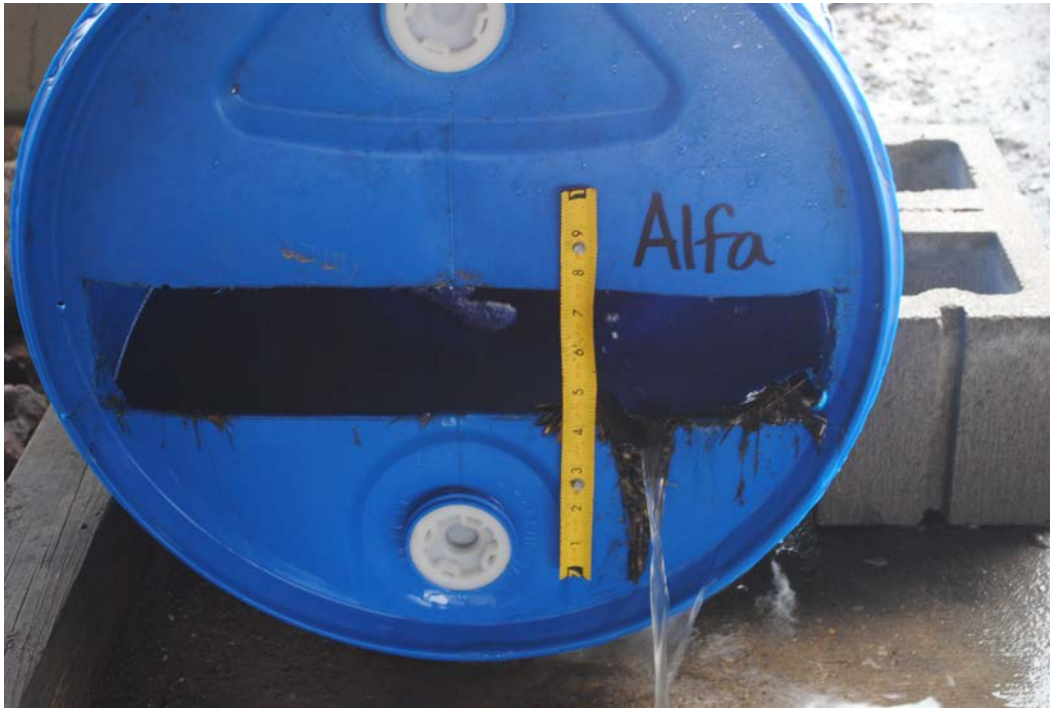
Figure 10. Debris clog at Location A, March 27, 2014.
