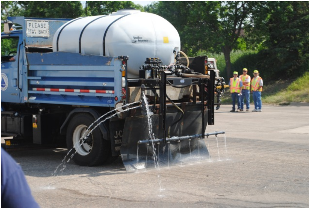
b) Brine application truck during demonstration (non-winter day).
