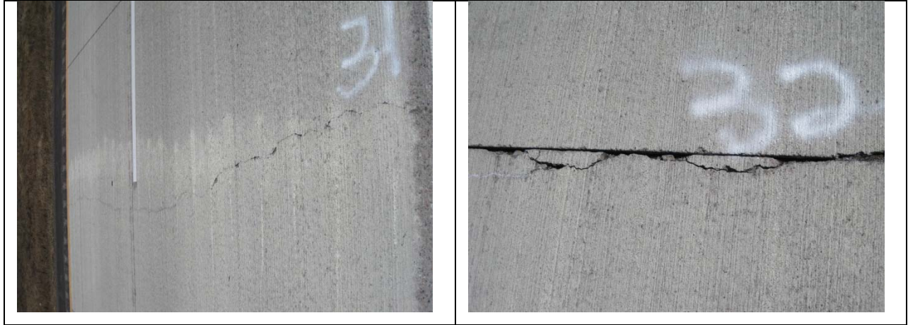
Figure A.16. Distress No. 31 [Left] & No. 32 [Right], April 2009
