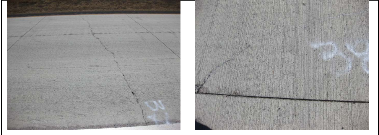
Figure A.19. Distress No. 37 [Left] & No. 38 [Right], April 2009
