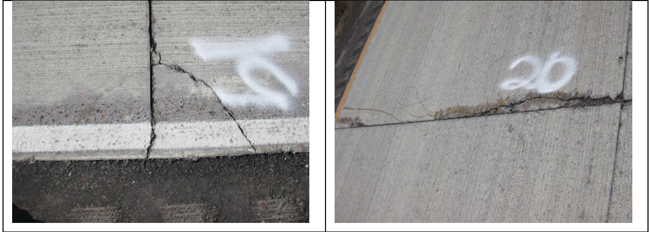
Figure A.10. Distress No. 19 [Left] & No. 20 [Right], April 2009
