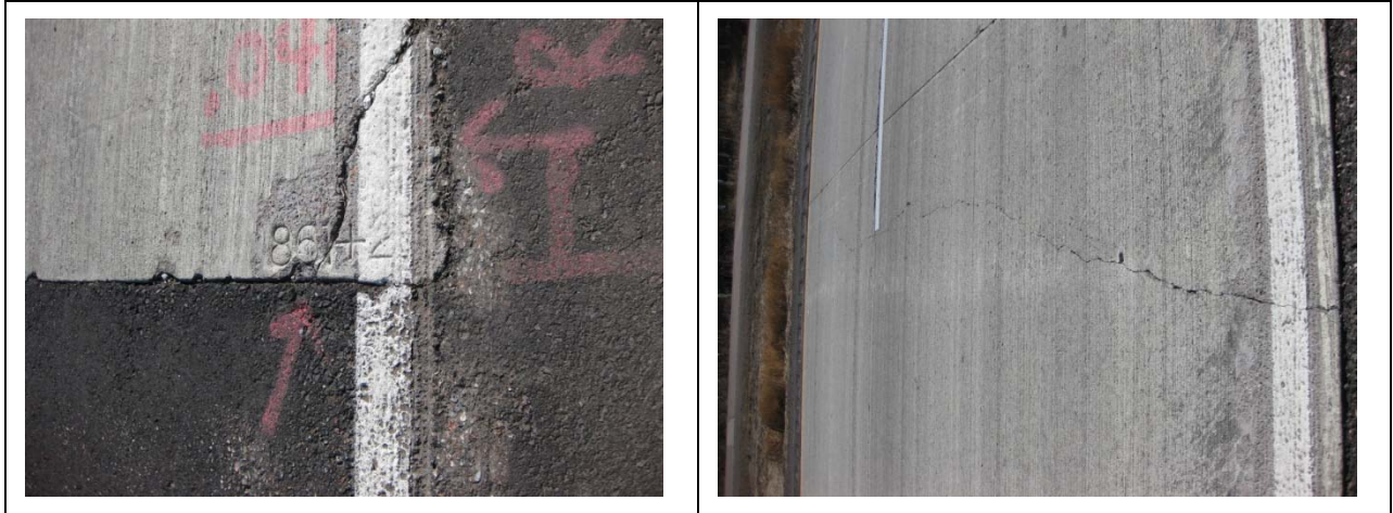
Figure A.1. Distress No. 1 [Left] & No. 2 [Right], April 2009
