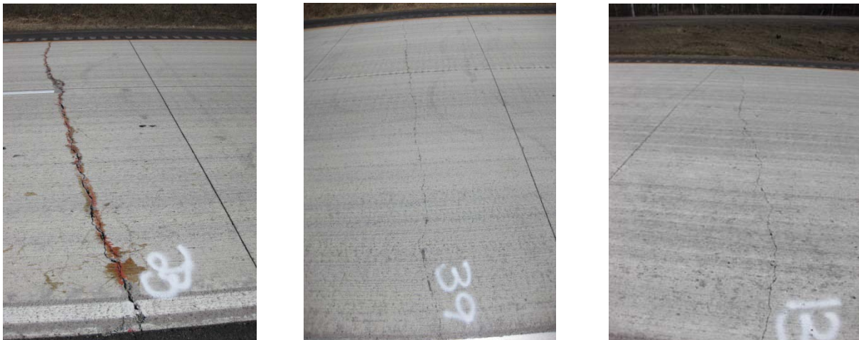
Figure 5.2. From Left to Right: High (3), Medium (2) and Low (1) Severity Cracking
