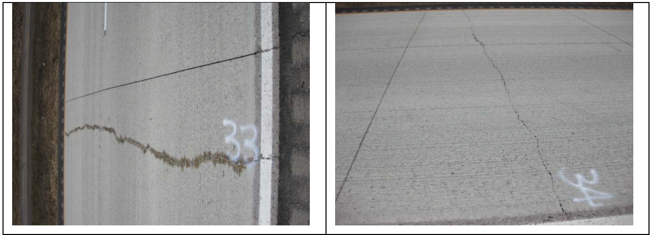
Figure A.17. Distress No. 33 [Left] & No. 34 [Right], April 2009
