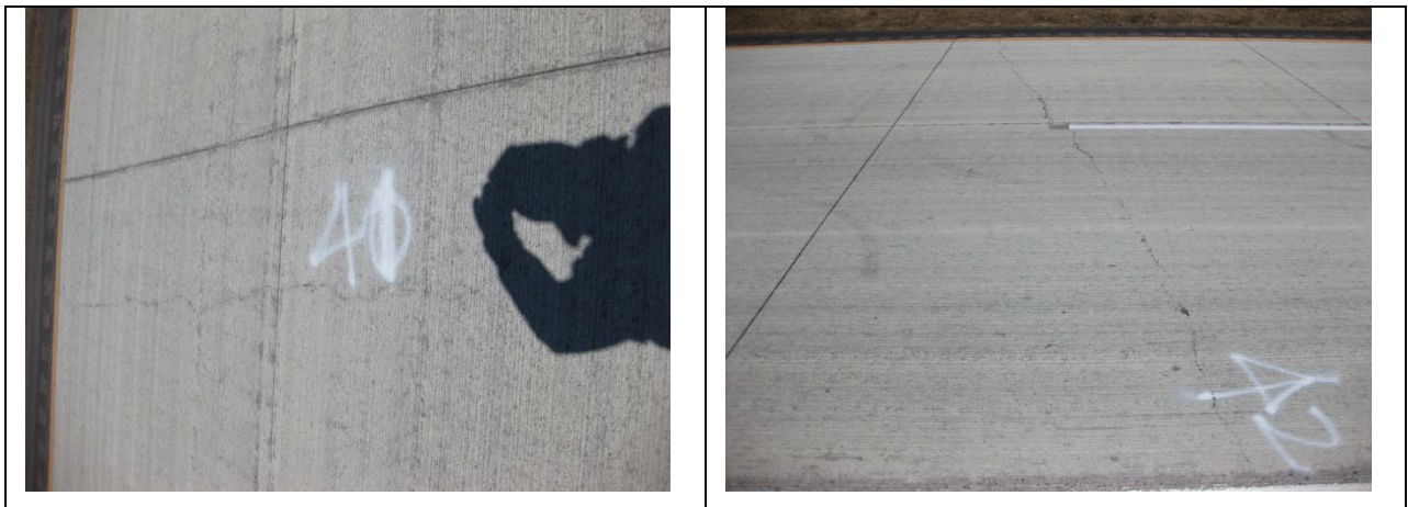
Figure A.21. Distress No. 41 [Left] & No. 42 [Right], April 2009
