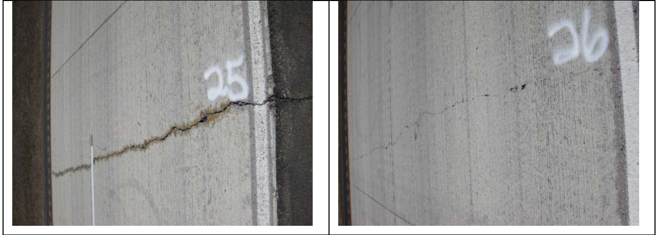
Figure A.13. Distress No. 25 [Left] & No. 26 [Right], April 2009
