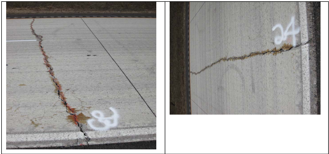
Figure A.12. Distress No. 23 [Left] & No. 24 [Right], April 2009
