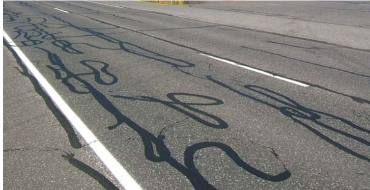
Figure 6: Excessive Crack Sealing
