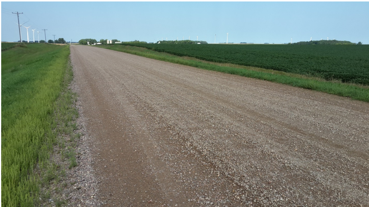
Figure 17. Jackson County CR 76 Surface Conditions in August 2013
