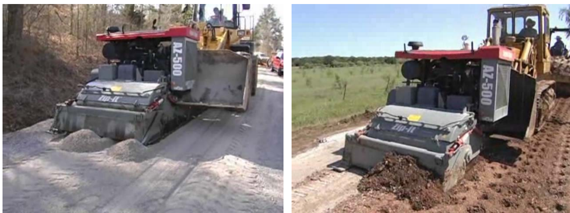
Figure 5. Asphalt Zipper in use for gravel road maintenance in Lafayette County, Mississippi (left) and Palo Pinto County, Texas (right) (Asphalt Zipper Inc. 2013a and 2013b)
