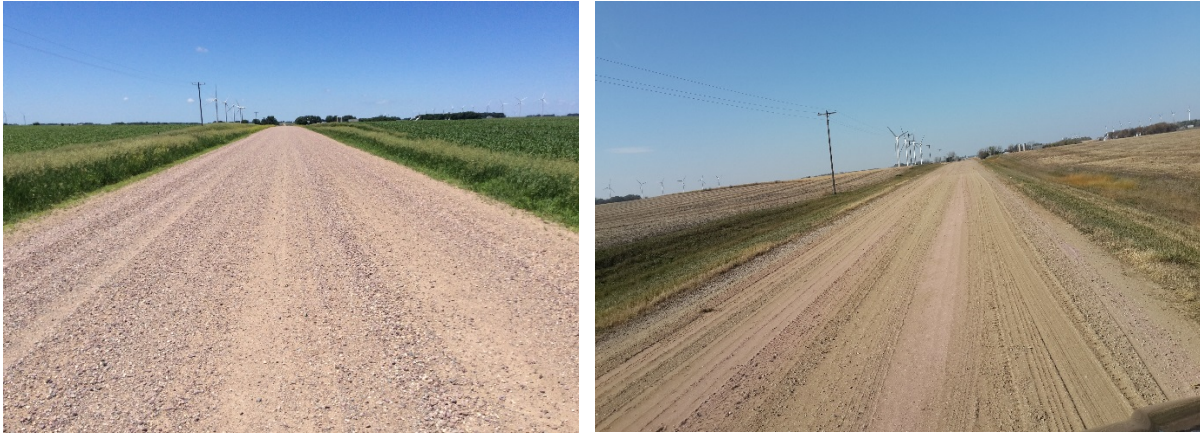
Figure 38. Jackson County CR 76 Seven Months after Construction
