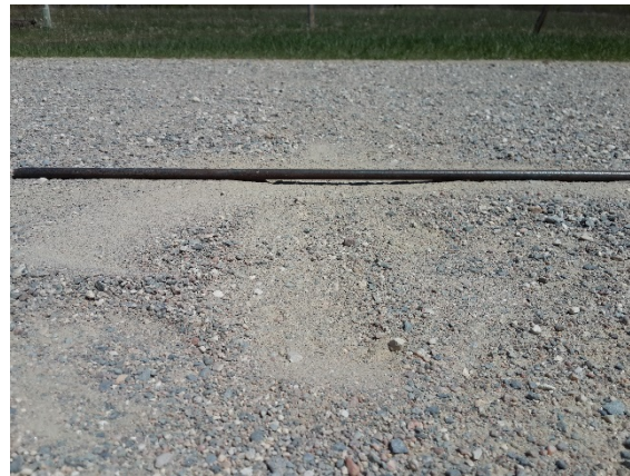
Figure 50. Typical Corrugation in the Beltrami County South/Third Test Section
