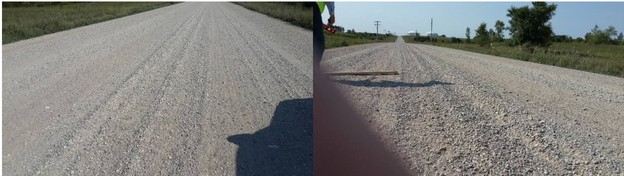
Figure 1. Excessive Floating Aggregate on Pope County CR 35 July 2013
