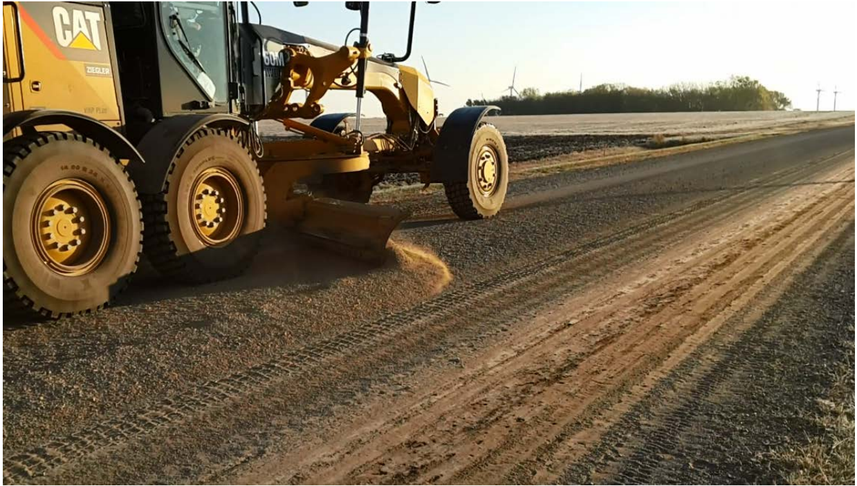
Figure 20. Windrowing Existing Loose Material in the Center of the Road at Jackson County Test Site
