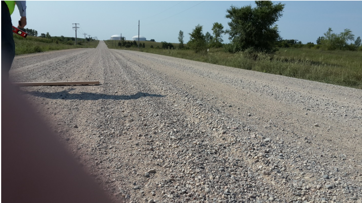
Figure 15 Floating Aggregate on CR 35 in Pope County
