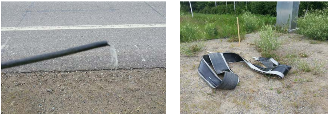
Figure 4-3: System after Vandalism
