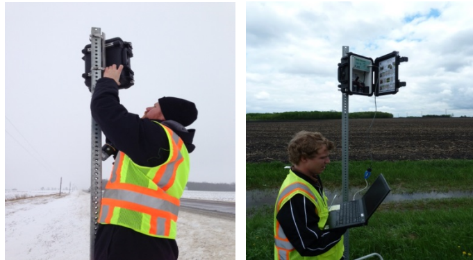
Radar Recorder Onsite Install and Configuration
