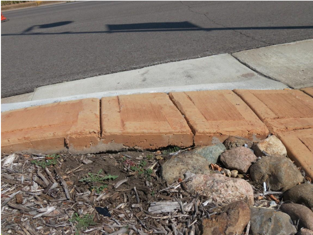
Figure 2.22 Brooklyn Center – Poor consolidation of boulevard along Bass Lake Road
