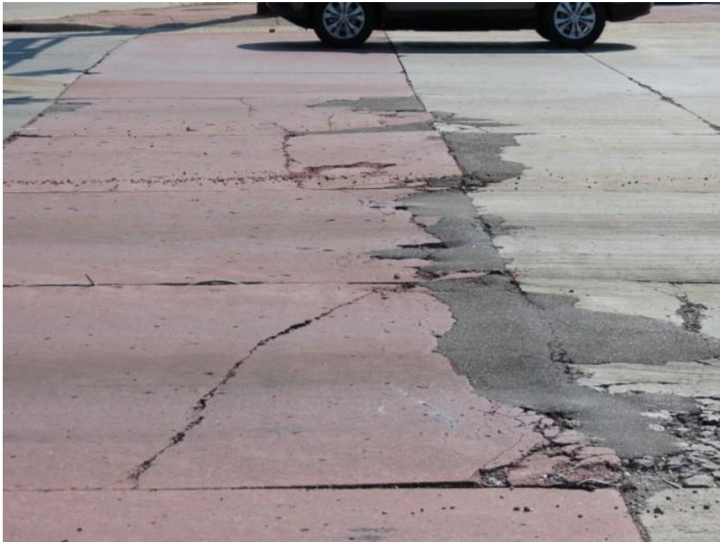
Figure 8.4 Deterioration of the slabs is too extensive, therefore requiring full slab replacement.
