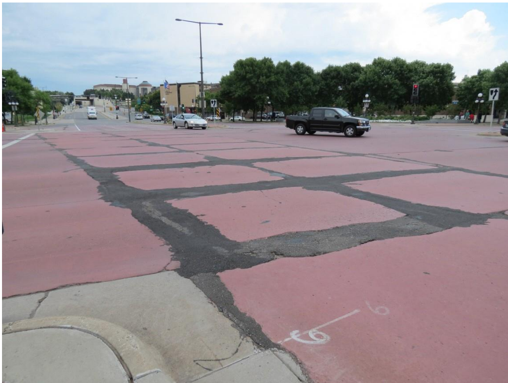
Figure 2.58 St. Paul – Widespread joint distress at intersection of 7th Street West and West 5th Street
