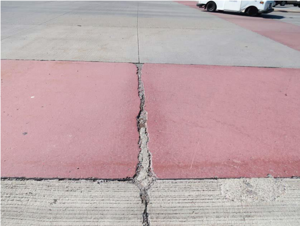
Figure 4.27 Typical joint deterioration occurring in colored concrete crosswalks at intersection of County Highway 96 and Greenhaven Drive in Vadnais Heights, MN
