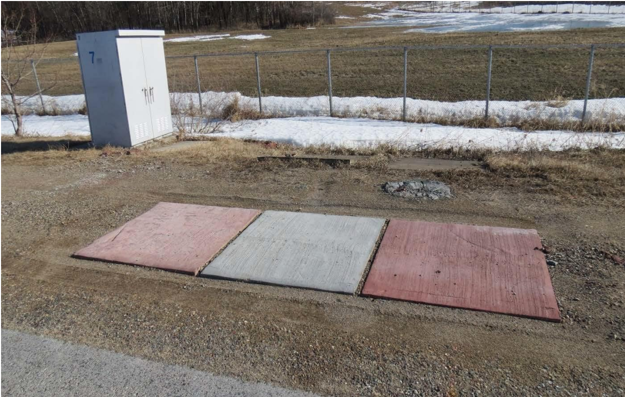
Figure 6.3 Concrete test slabs built at the MnROAD facility to evaluate the difference in thermal behavior under field conditions
