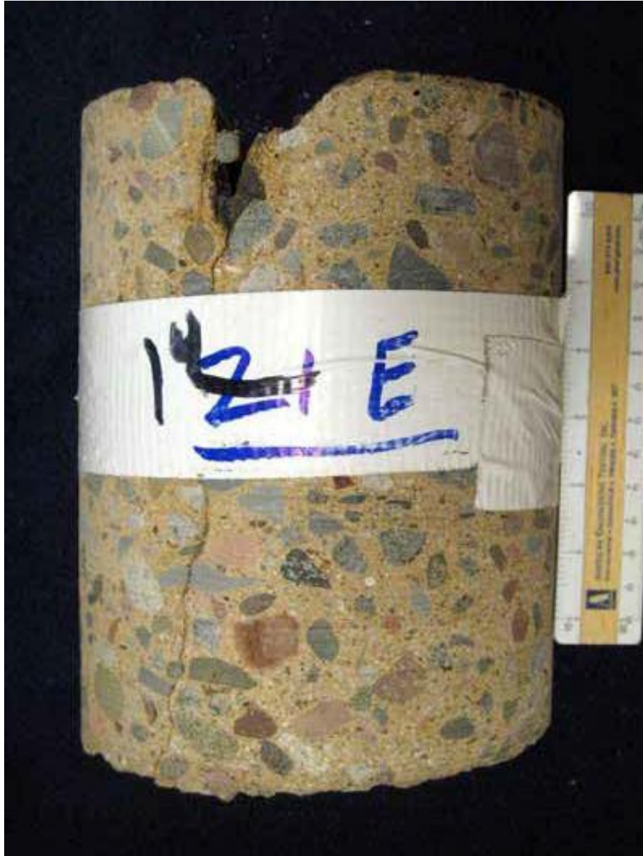
Figure 4.21 Centerville - Core 14E showing joint deterioration near surface
