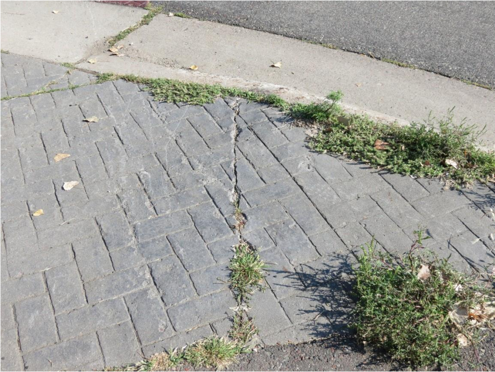
Figure 2.41 Roseville – Minor joint distress in colored concrete sidewalk near intersection of Josephine Road and Lexington Avenue
