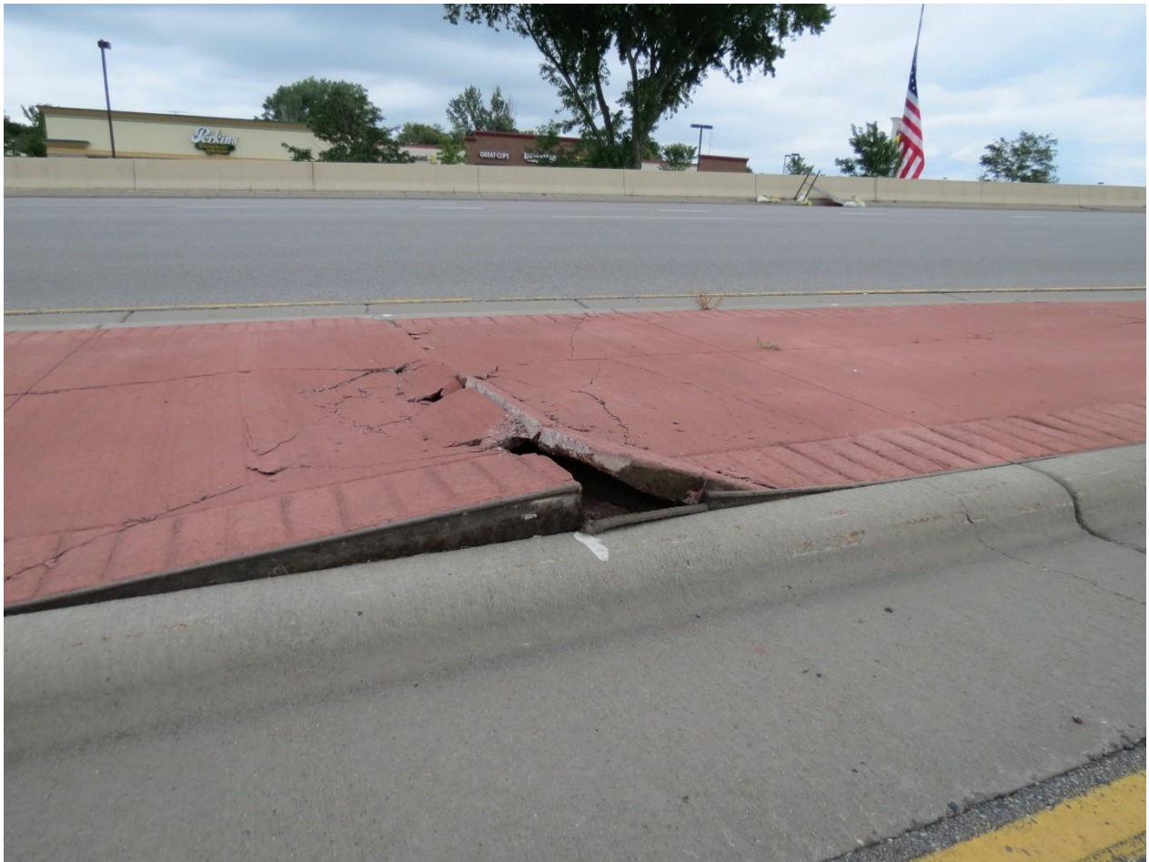
Figure 6.1 Buckled median caused by expansive forces in colored concrete
