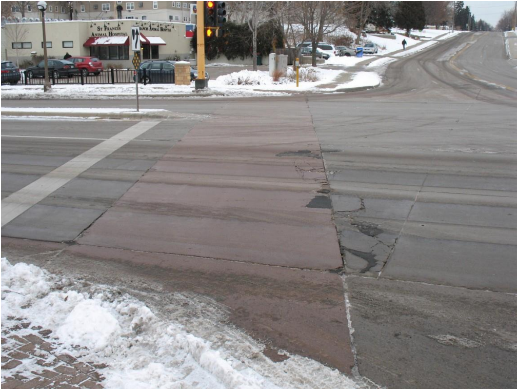
Figure 2.36 Roseville – Distressed areas in crosswalk panels at intersection of Larpenteur Avenue W and Fernwood Street
