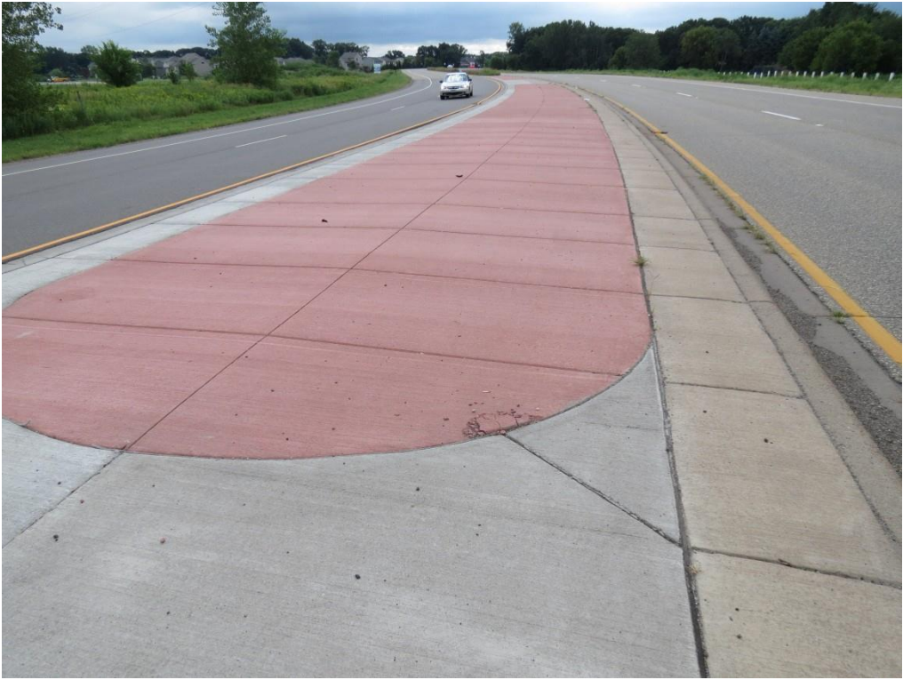
Figure 2.13 Blaine – Distress in median on Radisson Road
