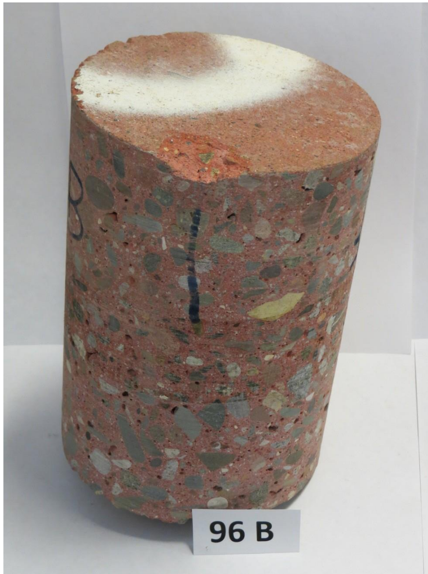
Figure 4.42 Vadnais Heights - Core 96B showing large number of air pockets throughout sample
