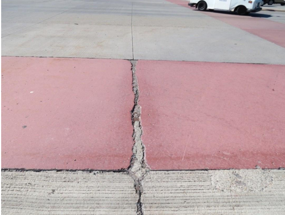
Figure 8.1 Example of joint distress in older pavement. Suitability for repair must be determined via core samples or other test methods.
