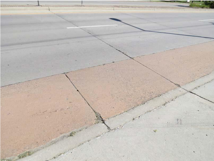
Figure 4.69 Distressed joints in parking lane along Larpenteur Avenue near Fernwood Street
