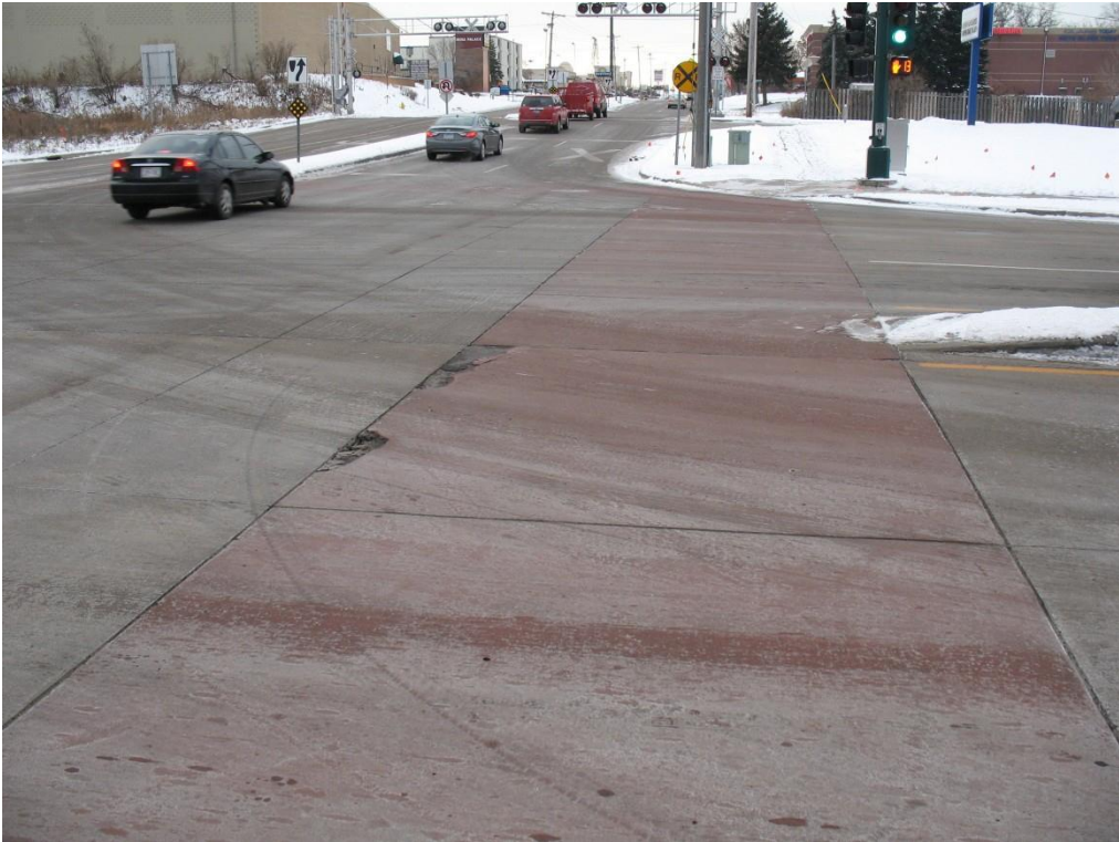
Figure 2.35 Roseville – Two distressed areas in crosswalk at intersection of County Road C and Cleveland Avenue N
