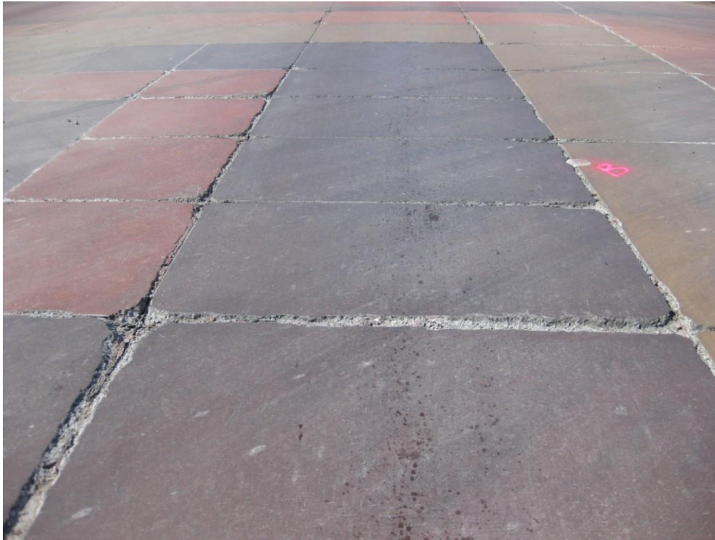
Figure 8.2 Example of joint distress in newer pavement. Suitability for repair must be determined via core samples or other test methods.
