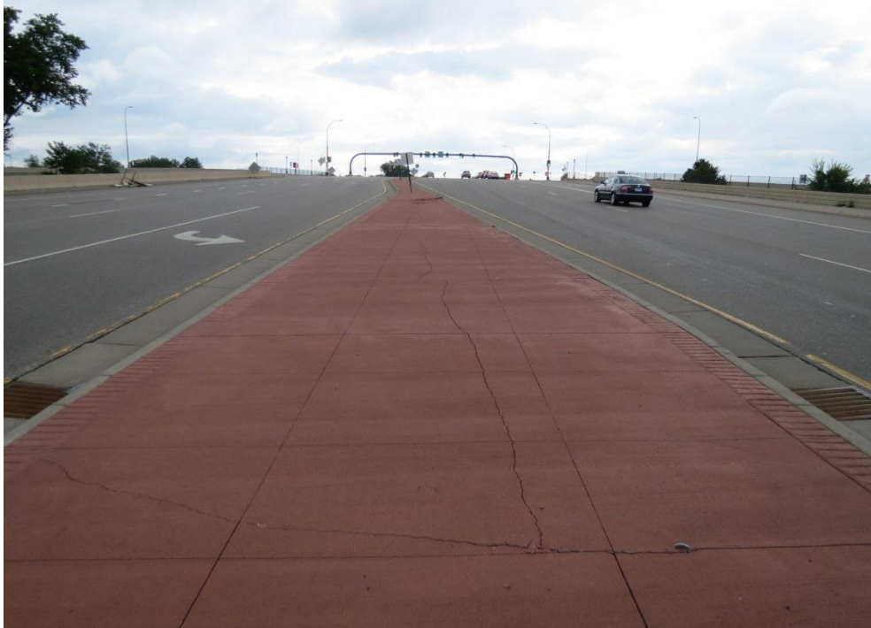
Figure 2.15 Blaine – Cracking of median within County Rd 14
