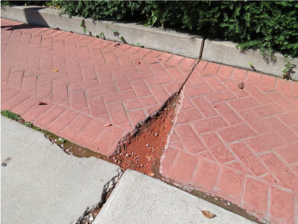
Figure 2.62 Stillwater – Significant joint distress in colored concrete sidewalks along 2 nd Street North between Myrtle Street East and Commercial Street
