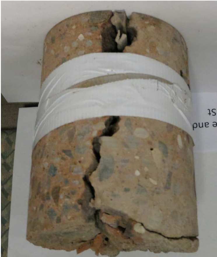
Figure 4.71 Roseville - Core sample L&F-A showing distresses at both top and bottom of joint
