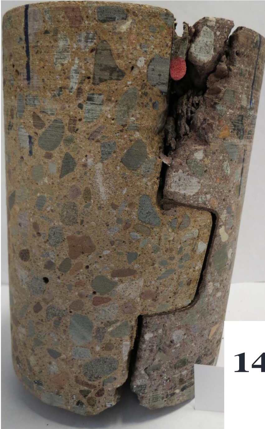
Figure 4.12 Centerville - Core 14B showing joint deterioration predominantly on side with darker concrete. Note that a parallel crack formed above the lower deterioration.
