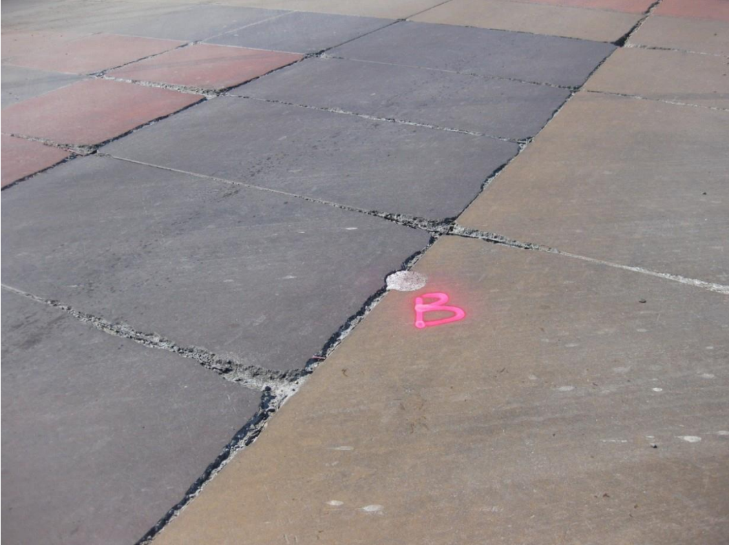
Figure 4.11 Centerville - Core location 14B, May 2013, showing progression of joint distress
