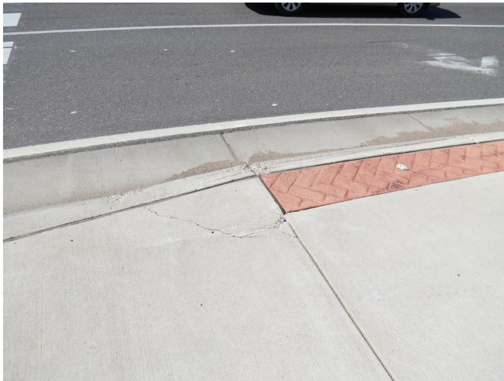
Figure 6.2 Crack in sidewalk, likely produced by expansion of neighboring colored concrete strip
