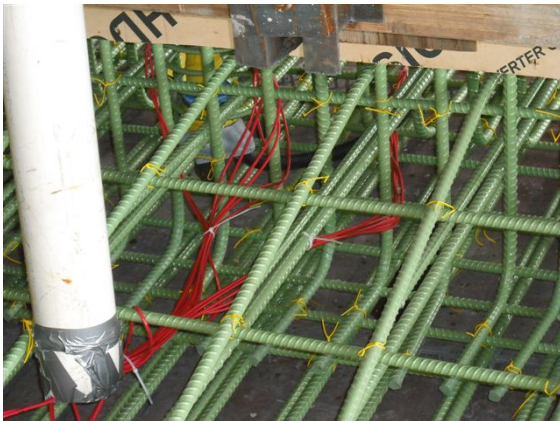
Fig A.4.5.1: Gauge leads in P4-6D are run to the PVC outlet pipe.
