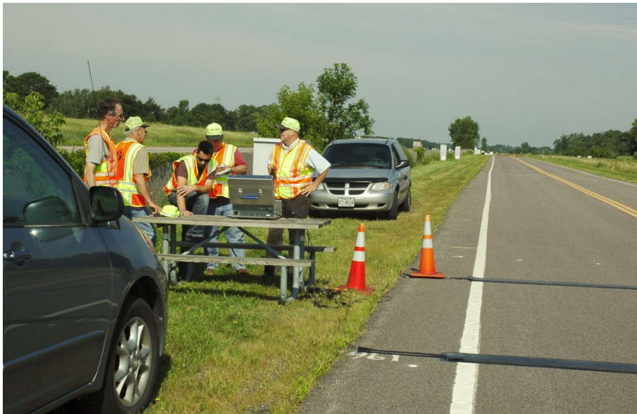
Nov 3 and 4, 2011, Cotton TH-53 Test. The top photograph shows an installation process of weigh-pads on TH-53. A temporary traffic control truck was called in, which can be seen in the back. The bottom picture shows the removal process of weigh-pads on the next day. The weigh-pad data was successfully collected for a side-by-side comparison with the IRD system in this site.
