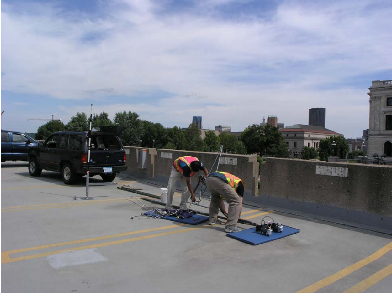
Figure E-3. Affixing camera mount platform to apex of camera boom, and preparing cable snake.
